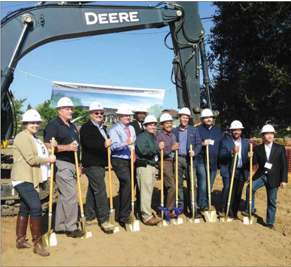
Management and development staff team up to launch the groundbreaking with the first dig. Photo by Paul Scholl
