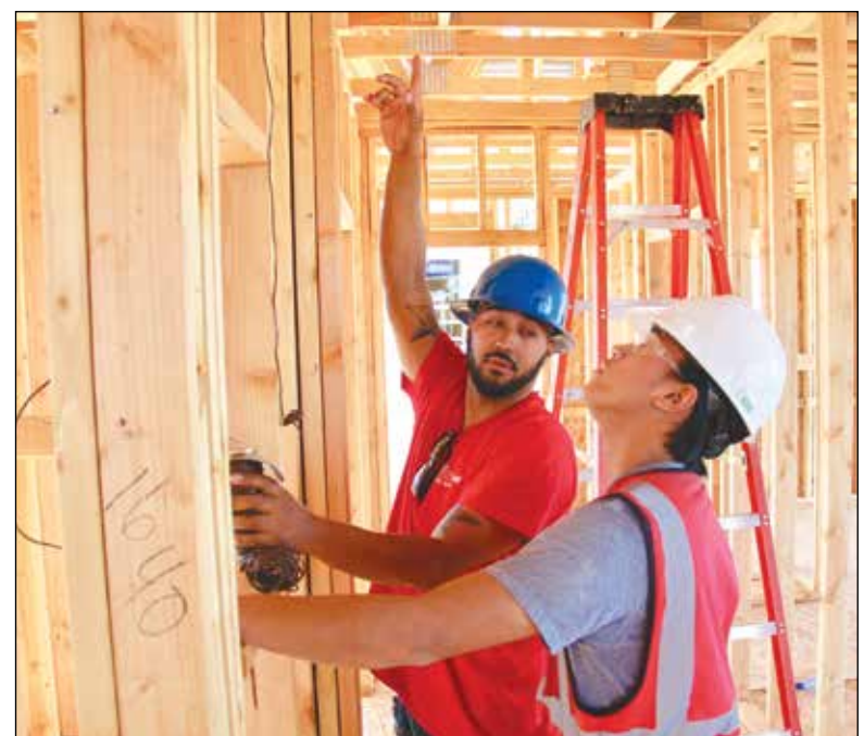
The program is a collaboration between the Foundation, major Sacramento-area homebuilders, a number of trade contractors, and 11 area high schools. (Above photo) Foreman Andrew Ruiz shows Jared Delacruz where the wiring will go in the attic.
