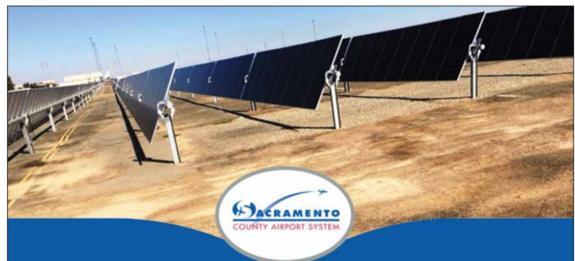
Energy company NRG owns and operates the airport solar facility and will sell electricity to Sacramento International Airport at below-market rates under a Power Purchase Agreement. Projected cost savings from the project are an average of $850,000 a year over the 25-year term of the agreement. Photo courtesy Sacramento County
