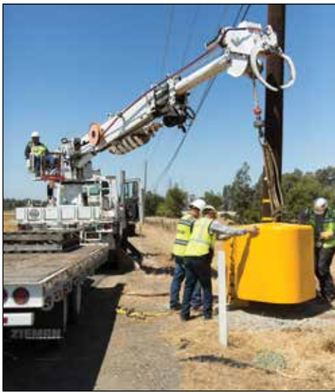
SMUD has installed some measures to mitigate damage to power poles and other electrical equipment by vehicles hitting them. The measures are part of a pilot program designed to increase visibility of and provide some protection to the power poles and to motorists. The work is part of SMUD's efforts to enhance public and worker safety and the SMUD grid's reliability. This photo shows a "Raptor" power pole barrier being installed in Wilton, CA. Photo courtesy SMUD
