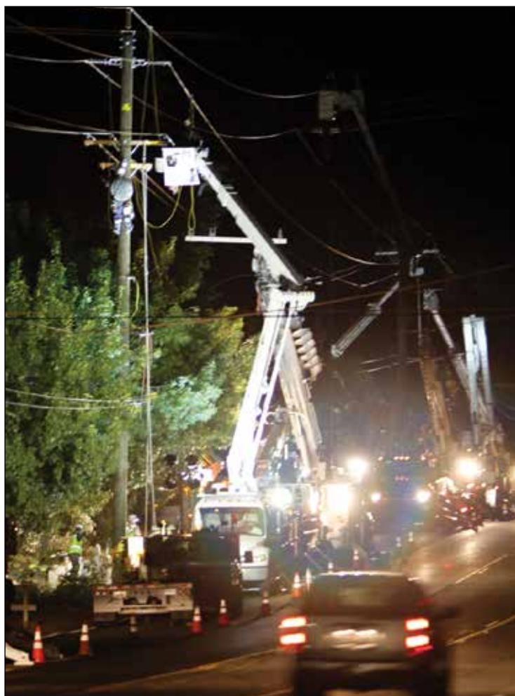
SMUD line crews replaced power poles on Hazel Avenue overnight June 28/29. The poles support 69,000-volt power lines that are the backbone of the SMUD system that delivers electricity to homes and businesses. The work is part of SMUD's efforts to enhance the SMUD grid's reliability.
