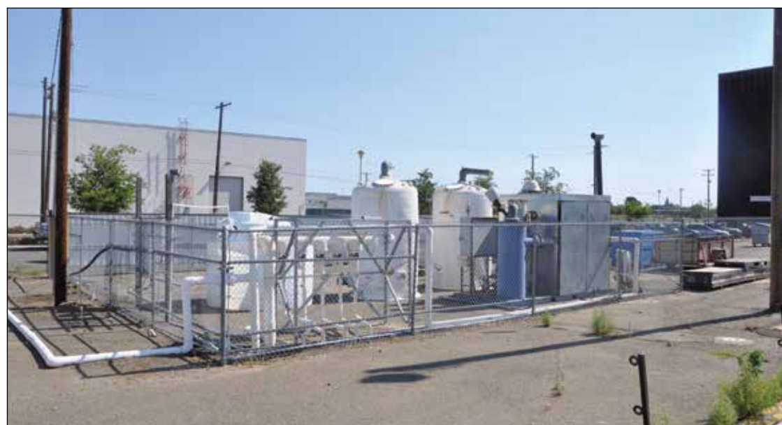
AFCEC's Soil Vapor Extraction unit, known as "Unit 59," cleaned this area once occupied by an airplane wash rack. This is one of several restoration systems at the former base that have removed 1 million pounds of volatile organic compounds and petroleum products from the ground and treated over 12 billion gallons of groundwater. Photo by Alex Grotewohl, AFCEC PA
