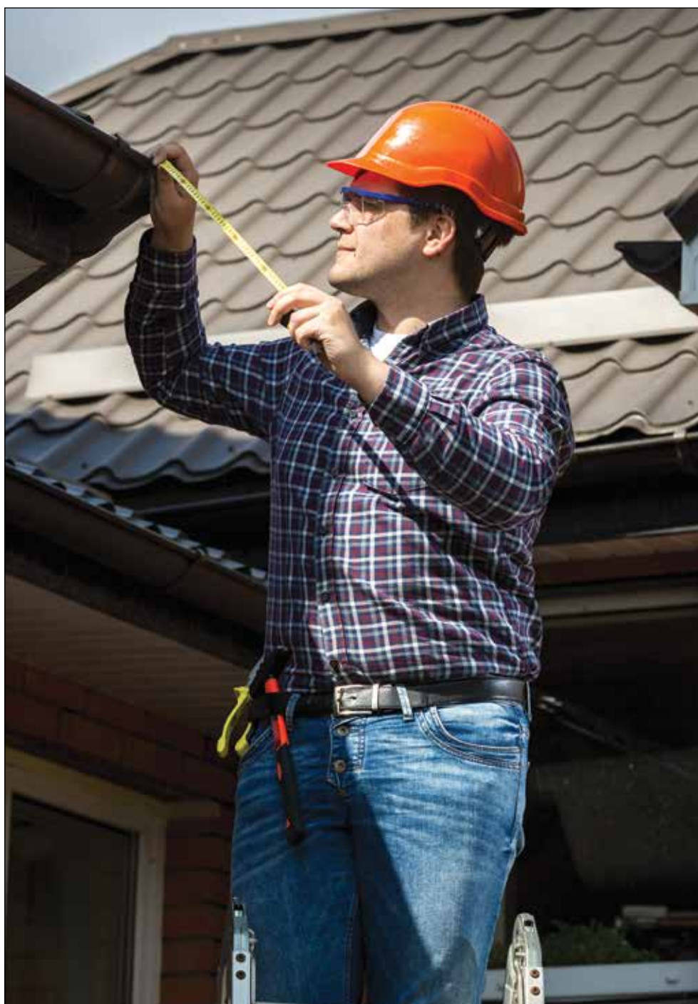
CSLB Tips Help Prevent Storm Repairs From Becoming Costly Headaches
