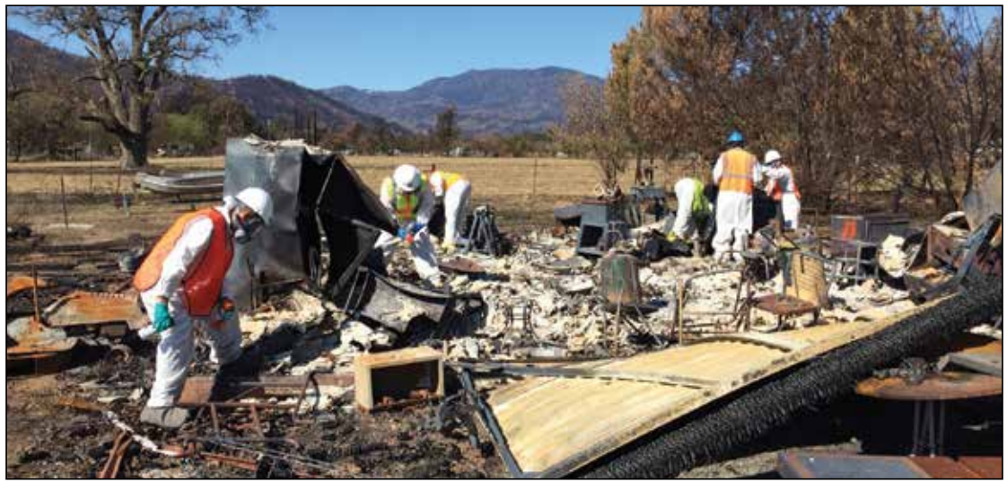
Valley Fire cleanup and debris assessment
