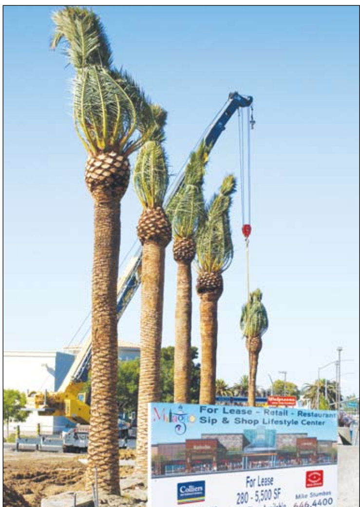
A delicate crane operation recently positioned massive Canary Island palms at the Milagro Centre on Fair Oaks Boulevard.
