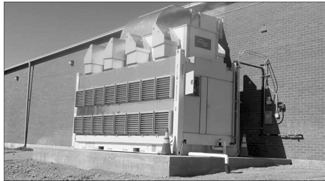
The Climate Wizard indirect evaporative cooling system helps Tri Tool, a large industrial facility in Rancho Cordova, keep cooling costs down. Climate Wizard is a type of "swamp cooler" that is very high performance, using 80 percent less energy than conventional industrial HVAC systems without adding any humidity.
