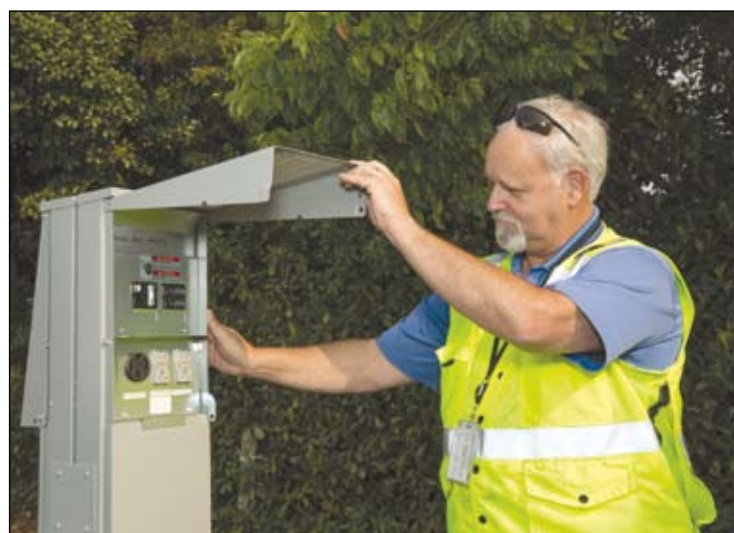
Sacramento Municipal Utility District (SMUD) Program Manager David Hatfield inspects newly installed "shore power" electric hookups at the Sacramento 49er Travel Plaza, a truck stop near the interchange of Interstates 80 and 5. By providing utility power where big-rig drivers spend their rest periods, truckers can plug in their rigs to electrical outlets and avoid idling their engines. By doing so, truckers save money and harmful emissions are reduced.
