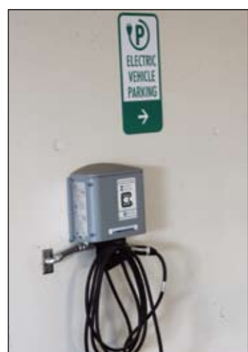
Electric charging stations such as this one at the new American River College parking structure sit empty most of the day. Photo by Mark Ahling
