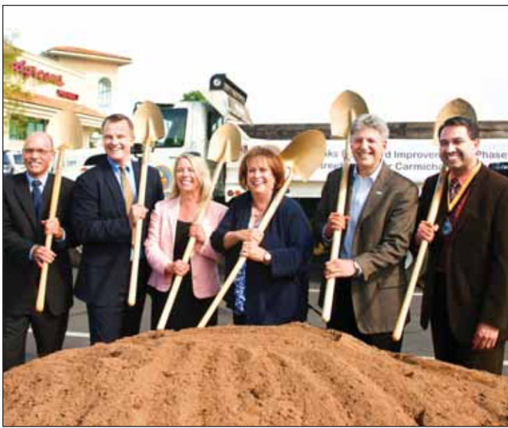
Community and County officials last week broke ground for the long awaited Fair Oaks Blvd Improvement Project. Digging in were: Transportation Director Mike Penrose (left), Carmichael Chamber of Commerce President Chris Meyer, County Planner Tricia Stevens, Supervisor Susan Peters, SMUD director Bill Slaton and honorary Mayor Esteban Nava. Photo by Susan Maxwell Skinner.
