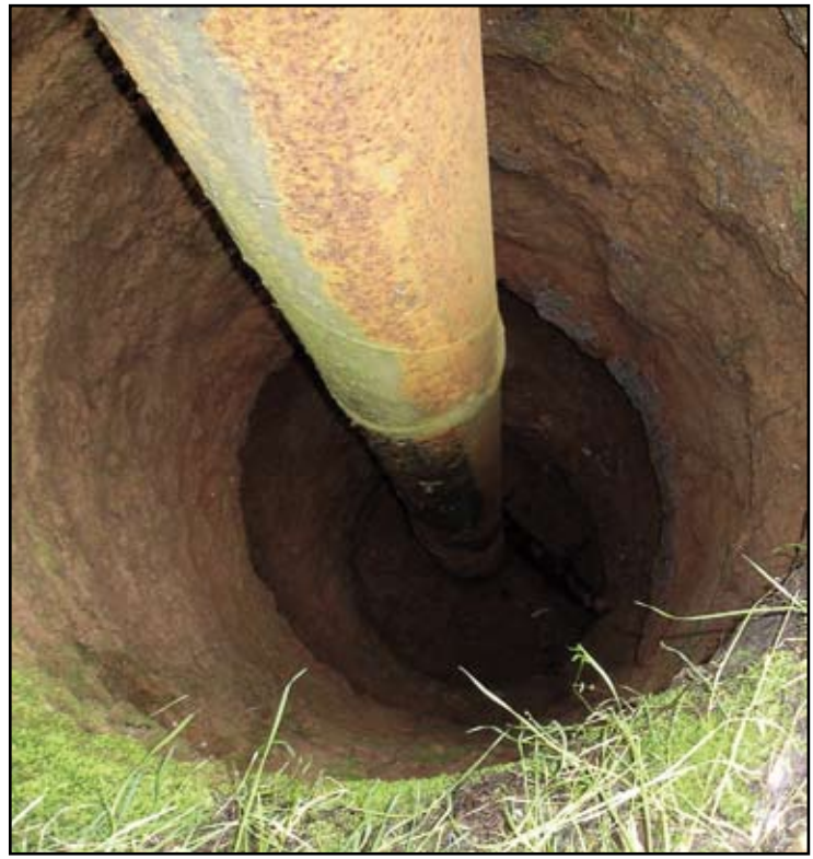
The Sacramento Region is dotted with abandoned wells such as this one, posing a hazard to residents. Photo courtesy of Sacramento County
