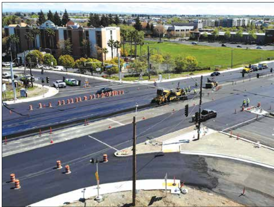
Road work continues in Rancho Cordova, aided by the decrease in traffic. Photo Courtesy City of Rancho Cordova
