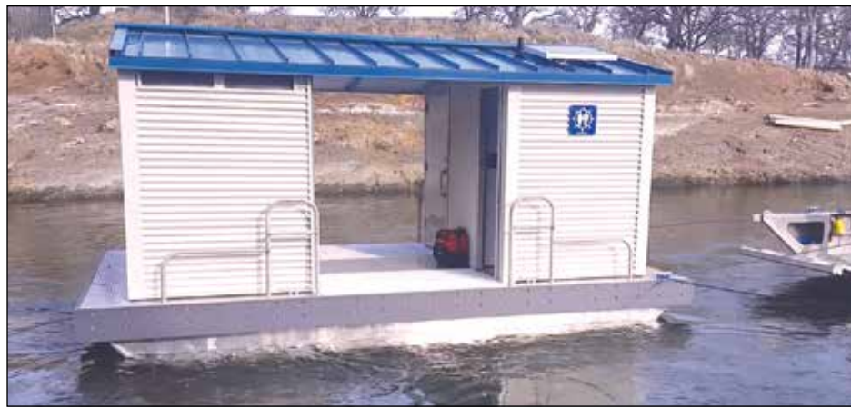
Floating restroom shown during December 2019 deployment at Lake Berryessa. Each ADA compliant unit holds about 500 gallons of sewage. Photo courtesy California State Parks
