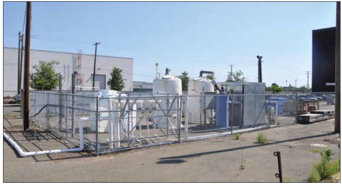
AFCEC's Soil Vapor Extraction unit, known as "Unit 59," cleaned this area once occupied by an airplane wash rack. This is one of several restoration systems at the former base that have removed 1 million pounds of volatile organic compounds and petroleum products from the ground and treated over 12 billion gallons of groundwater. Photo by Alex Grotewohl, AFCEC PA
