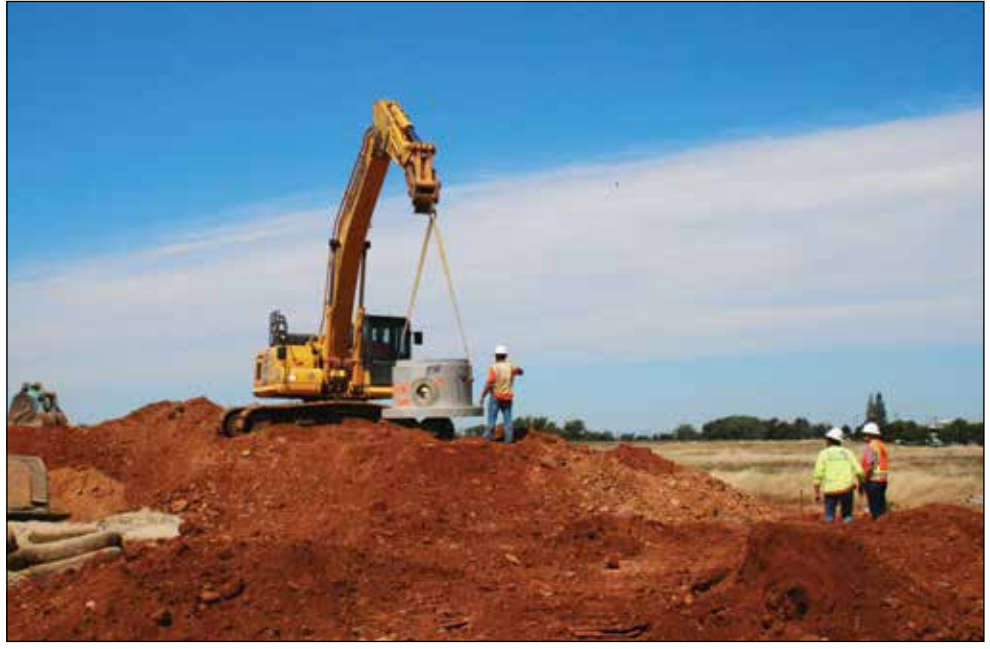
Workers are currently installing drainage tiles at the new Raley's complex on the southwest corner of Sunrise Boulevard and Douglas Boulevard in Rancho Cordova. The projected date for the grand opening of the complex is sometime in mid 2017.
