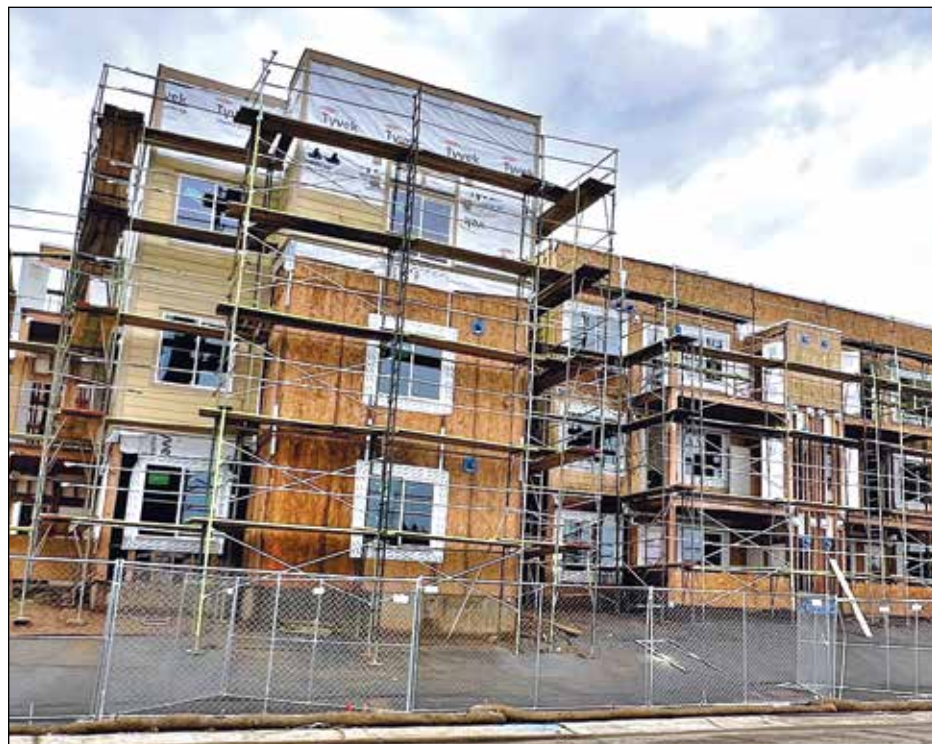
The Cemo Circle apartment complex under construction should be a boon to the adjacent tenants of Village Marketplace. Photo by David Dickstein
