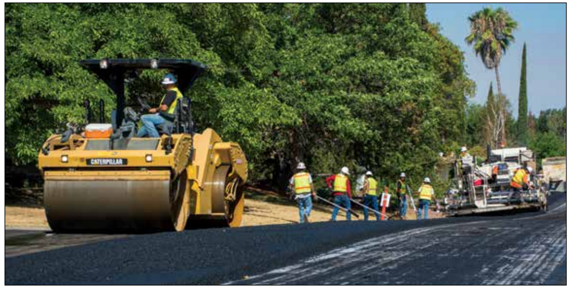
Seeno Road repaving in Granite Bay. Photo courtesy of County of Placer
