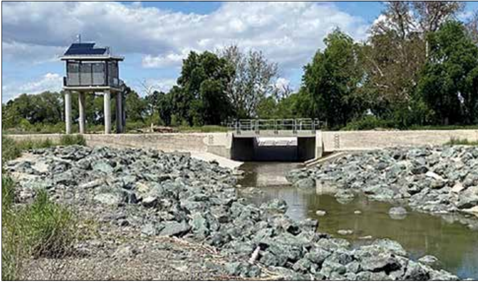
This is the second year the Fremont Weir Adult Fish Passage has operated. Due to drought conditions, the facility was last operated in the winter of 2019. Photo courtesy of DWR.
