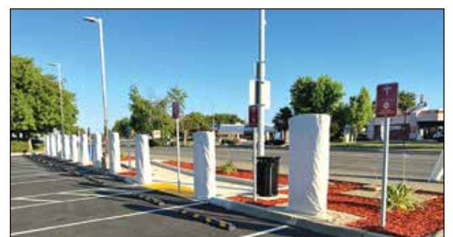
Twelve Tesla Charging Stations have been installed in the Safeway Shopping Center and appear ready but have not been released for use yet.
