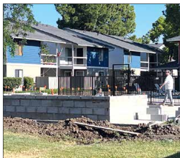
A man walks by the construction area for a new barbecue area at the large apartment complex on Pitt School Road and H Street.
