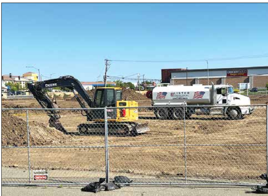
The Bank of Stockton project, which was approved in early 2022 is now being built out at the corner of North First Street and Vaughn across from Grocery Outlet and next to Tractor Supply. There will also be two separate retail buildings, which would host retail, food or drive-thrus (no tenants or specific uses identified early 2022 for those buildings,) according to Raffi Boloyan, City of Dixon Community Development Director. Photo by Debra Dingman
