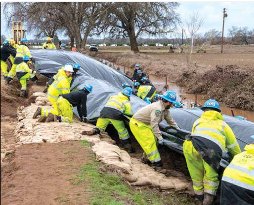
Another dangerous storm is barreling toward the Sacramento Valley, where rains already punched through some levees. Photo courtesy of DWR
