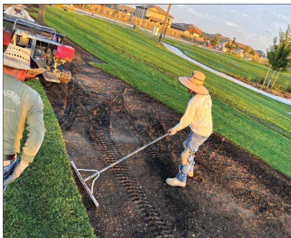
Large 3-foot by 3-foot spools of turf were unfurled on top of fertilized and prepared sod by small tractors at the new Southwest Park on Pitt School Road last week during the heatwave. Several workers who were arranged through Southwest developers packed it snugly into place. Dozens of sprinklers twirled water to keep the new grass moist so that it would take root and be ready in approximately a month for children to be able to play on if the new grass is approved by the City of Dixon. Photo by Debra Dingman
