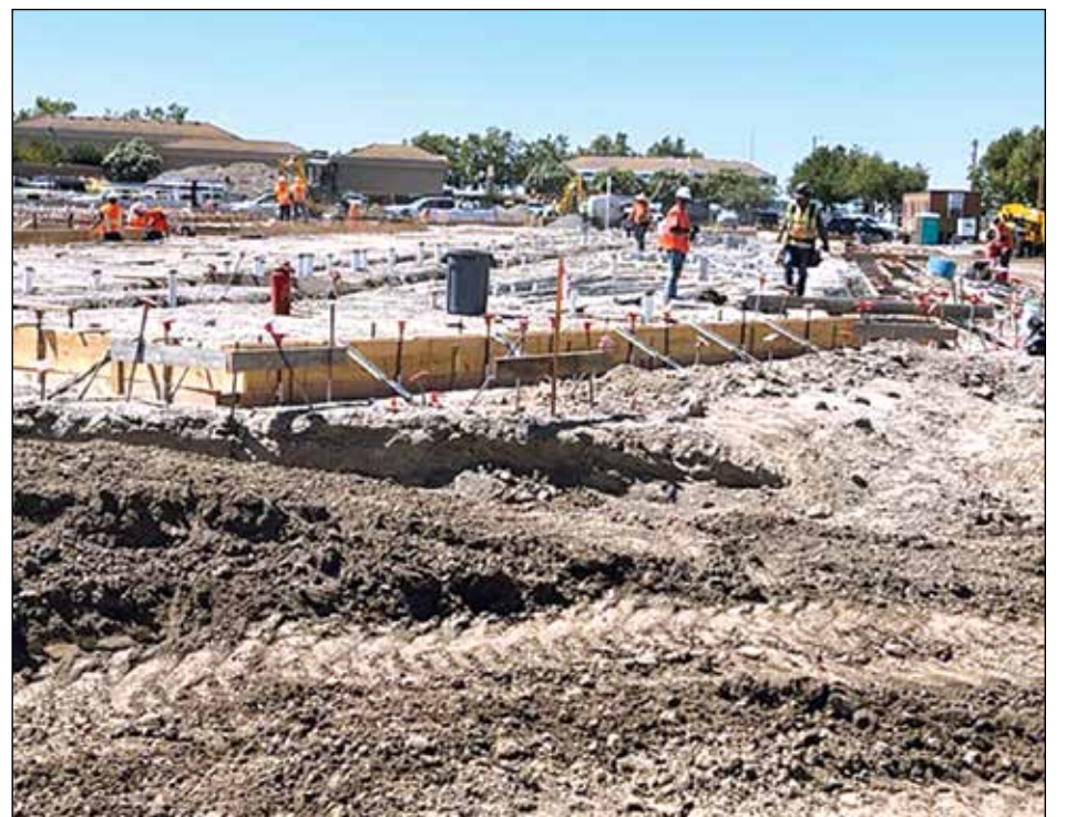
Numerous workers and lots of equipment working on the foundations of the senior living facility being built on Gateway Boulevard
