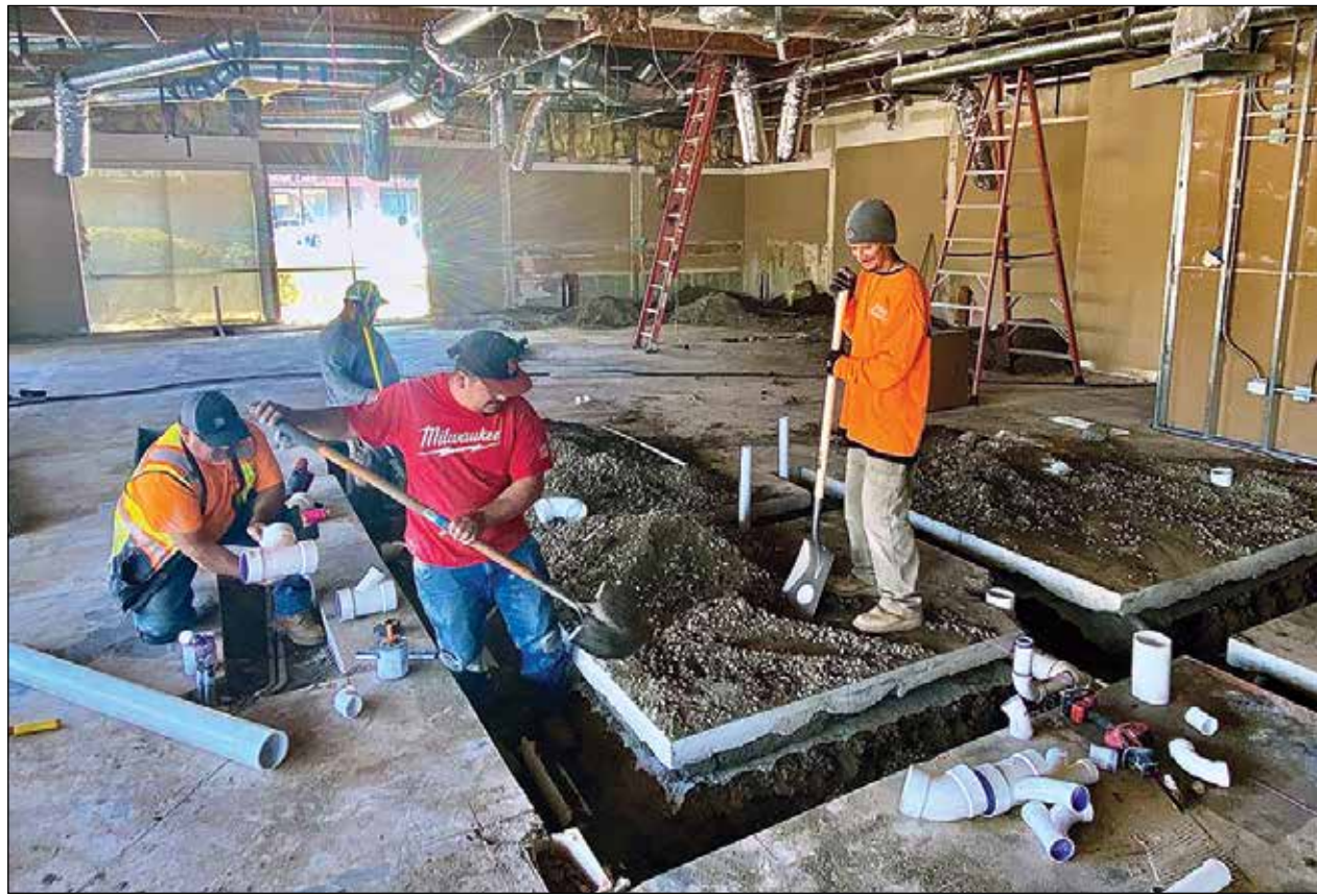
This construction crew is working on the new foundation of the NorthBay Urgent Care Center which is in the Safeway Shopping Center, formerly the Chase Bank building. Photo by Nicolas Brown
