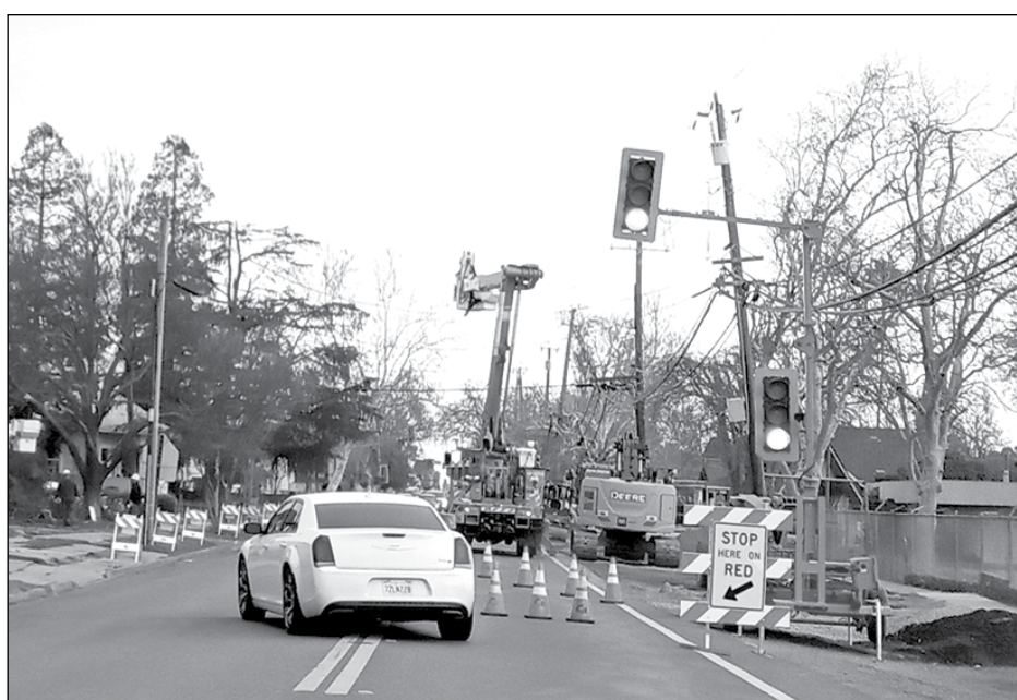
Expect a few more days of traffic delays on Highway 113. The work at the South First Street and Chestnut intersection as well as the South First Street and Valley Glen intersection includes traffic signal installation and associated public improvements, according to the City of Dixon. Work specific to the Chestnut intersection is storm drain piping improvements, traffic signal installation, and roadway resurfacing to accommodate new ADA ramps and crosswalks. Photo by Debra Dingman
