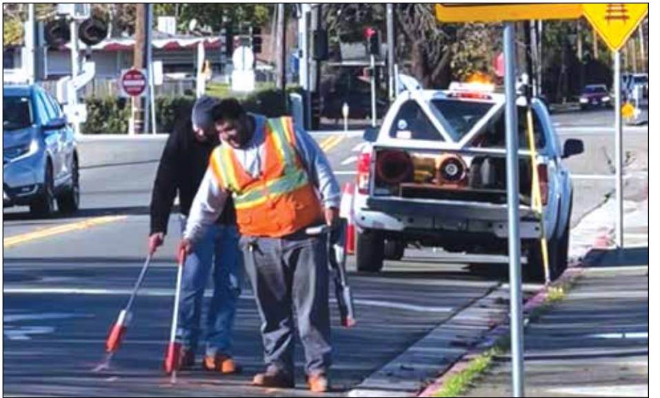
These workers are marking the road along West A Street for future construction of a new gas pipe, they said. They note where all the other utilities are underneath so they are not damaged when digging begins. Photo by Debra Dingman
