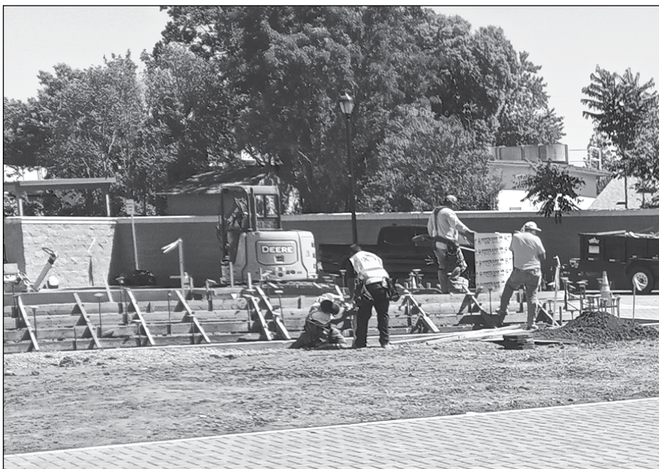
Work continues behind the scenes at the Pardi Market Plaza at the corner of A and First Streets with construction of the stage being part of Phase 2. Downtown visitors are finding parking spots elsewhere but not happily as they saw concrete and bark torn up that had just been put down about a year ago in Phase I. The new construction is supposed to be done in November. Photo by Debra Dingman
