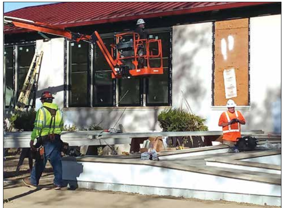
Work continues with the installation of new windows at the old Dixon High School that is becoming the new John Knight Middle School. This is one of the last things to do, according to Melissa Maseda, Dixon Unified School District Oversight Committee Member. The building renovations are being completed with the exception of the kitchen so "teachers are packing boxes now" and will start moving in over the Winter Break, she said. When school starts in January, they should be in place. The kitchen has a lot more work to be done in order to meet code requirements so students will have to bag lunch - when and if students can return physically to campus in the new year. Photo by Debra Dingman
