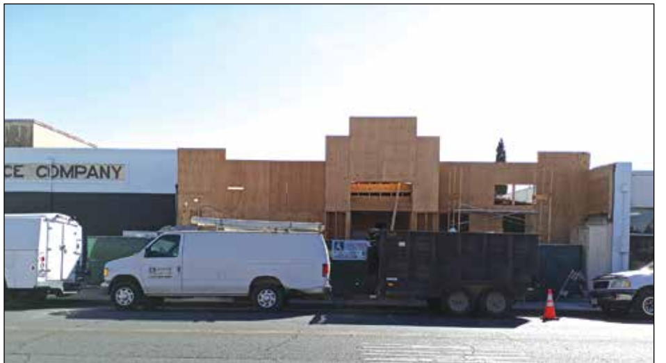
Ascher Properties is working daily on the facade improvement of the Community Medical Center at 131 West A Street in downtown Dixon. The medical center has been a major tenant for two decades but began as a volunteer effort in the 1960s. They offer Family Practice, Health Education, Nutritional Counseling/Dietitian, Perinatal - CPSP Behavioral Health, Quest Laboratory, Diagnostic Laboratory, Outreach & Enrollment, EIS/HIV Testing, Screening and more. Every day, their staff provides vital care to men, women and children, regardless of ability to pay. Ascher and his crew expect to be finished by the end of November. Photo by Debra Dingman
