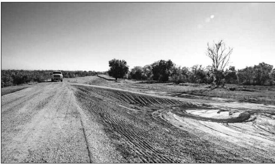
The recently-completed Bear River Setback Levee in Yuba County. Photo courtesy of Yuba Water Agency
