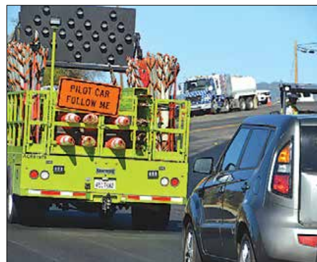
Construction crews will be conducting reversing, one-way traffic control during daylight hours at various times and locations between Marysville Road and the Parks Bar Bridge at the Yuba River. Photo courtesy of Caltrans
