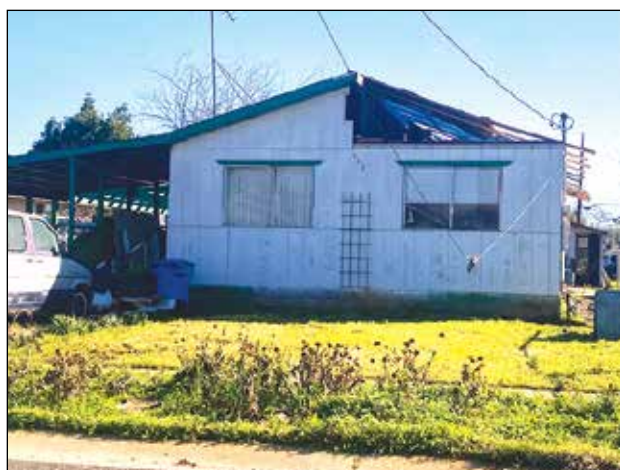
The 3 realtors could see from the street that the Tulip Lady's house was open to the elements. Photo: EXP Realty of California
