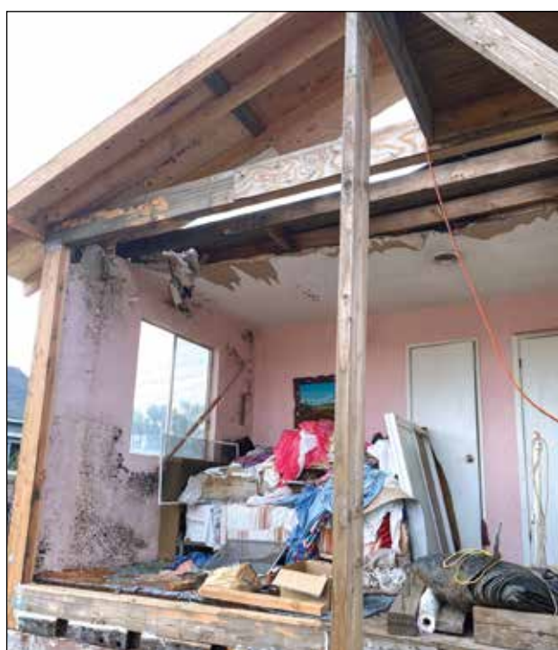
Construction material including insulation and sheetrock littered the inside of the house. Photo: EXP Realty of California
