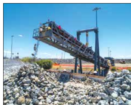
Rock is loaded onto barges at the California Department of Water Resources Weber Rock Yard near the Port of Stockton, California. The purpose of the rock barrier is to prevent the Delta from becoming too salty for irrigation, drinking water, or fish. Photo by Florence Low/California Department of Water Resources
