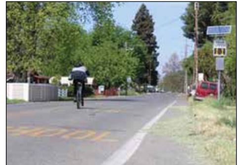
The project includes West Linda’s first-ever curb, gutter, and sidewalk along surrounding streets – including Alicia Avenue, pictured here with – construction expected to start this spring. Photo: Yuba County
