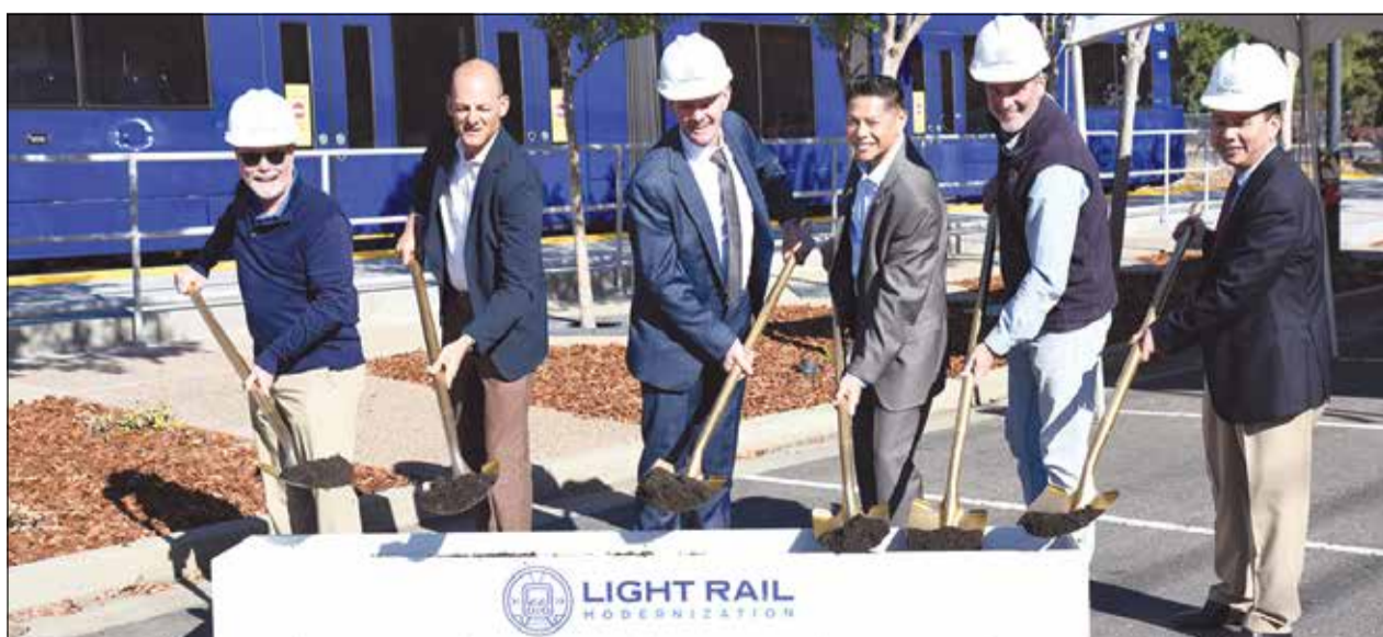
Groundbreaking ceremony at Iron Point Station on Wednesday, November 8, 2023, which will connect Folsom with 15-minute light rail services. From left to right: SacRT Board Chair and Sacramento County Supervisor Patrick Kennedy, Assemblymember Kevin McCarty, Michael Cahill, President of Siemens Mobility in North America, Darren Suen, Chief of Staff for Assemblymember Stephanie Nguyen and Elk Grove Councilmember, Mike Kozlowski, SacRT Board Director and Folsom City Councilmember, and SacRT General Manager/CEO Henry Li. Photo courtesy of SacRT
