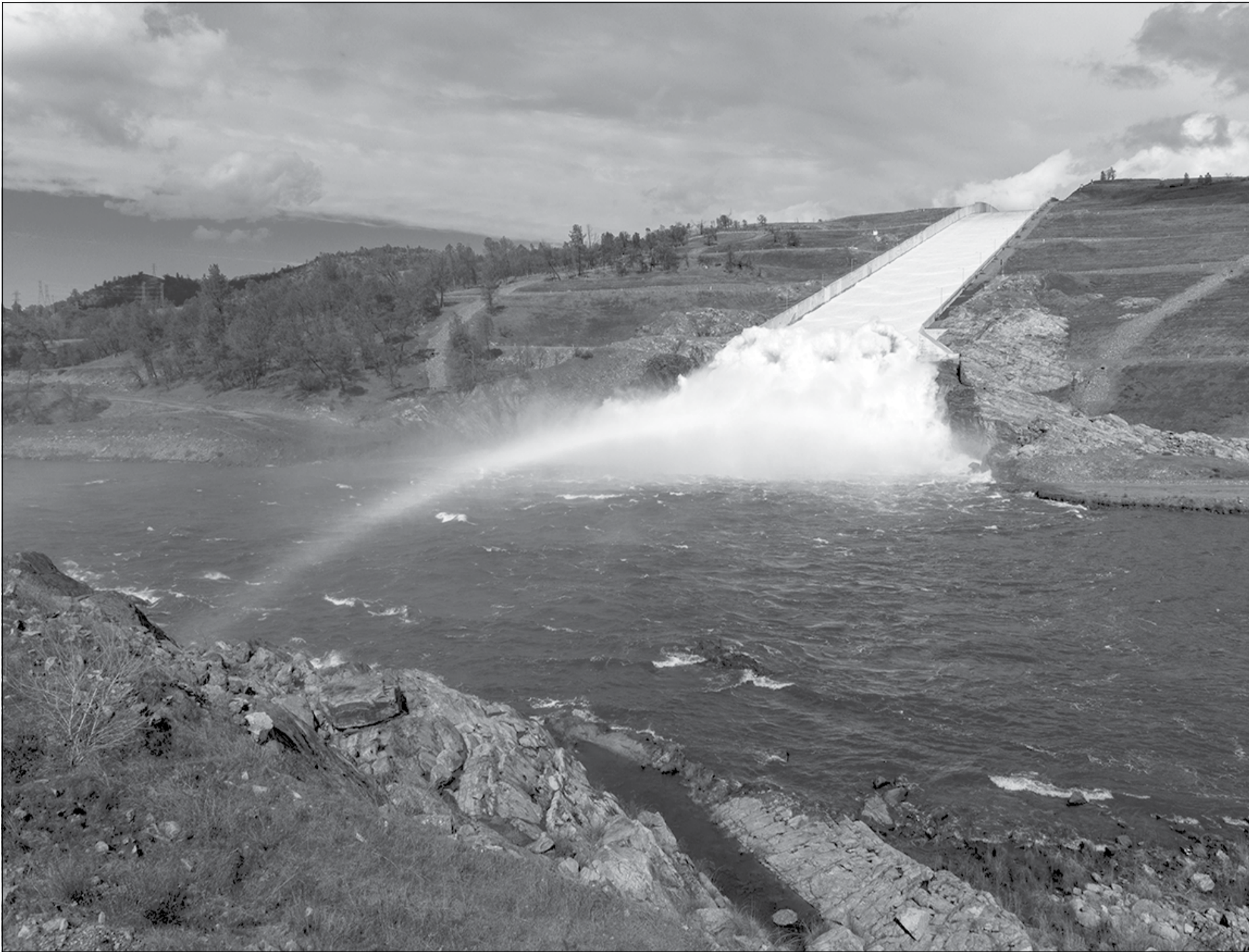
Storms have arrived in California. The Oroville Spillway at Lake Oroville in Butte County is ready for a wet year. California Department of Water Resources
