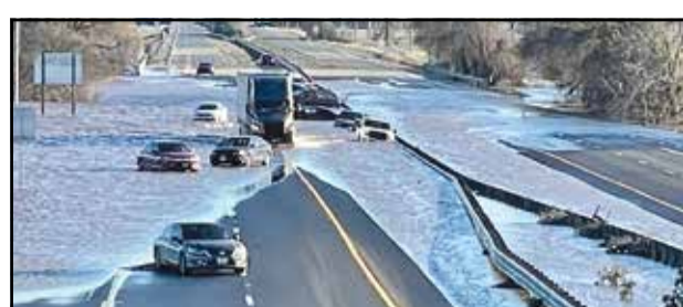
Flooding on Highway 99 at Dillard overpass last winter. MPG Courtesy Photo
