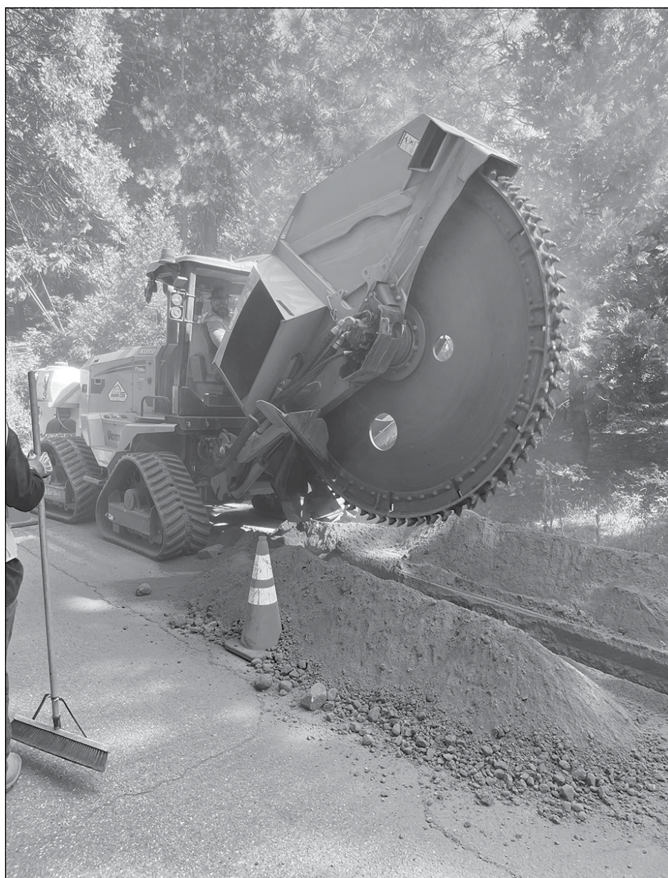
A rock wheel trencher is used by PG&E for some undergrounding projects. Photo courtesy of PG&E
