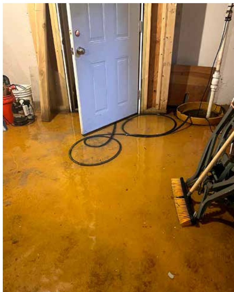
Mendon resident Shannon Hurley's basement experienced severe flooding in 2021, but there have been no issues since installing French drains and sump pumps. Photo courtesy of Shannon Hurley
