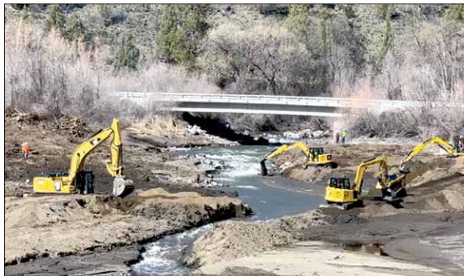
KRRC contractors dumping hundreds of tons of polluting sediments into Jenny Creek, which empties into the Klamath River. Photo: Bieke Lieckens
