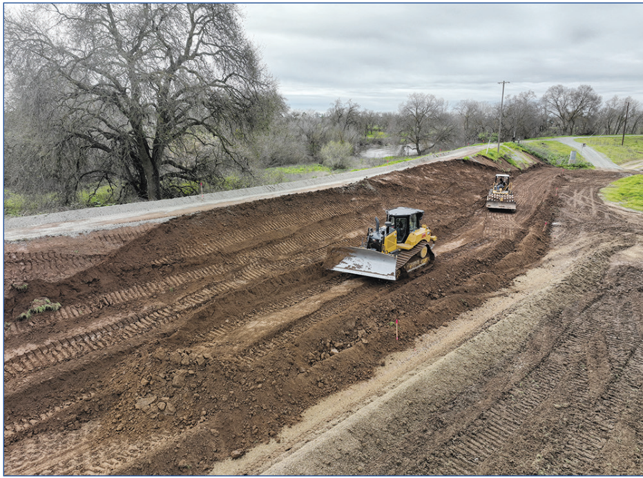
An aerial image shows emergency levee repairs at the end of Bradley Ranch Road in Sheldon after a high-water event on March 2. Courtesy photo
