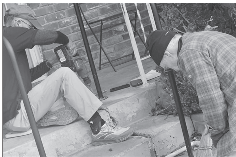
Safe at Home volunteers Dan Ward, of Carmichael, and Stan Jones, of the Greenhaven/Pocket area, install a handrail for a Sacramento resident in need of safer step way. Photos courtesy of SAFE Credit Union
