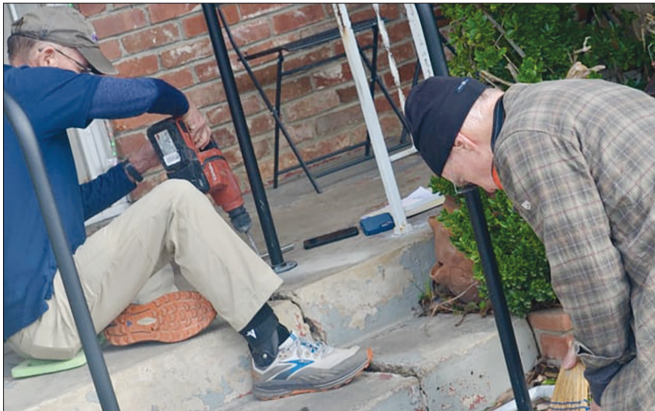
Safe at Home volunteers Dan Ward, of Carmichael, and Stan Jones, of the Greenhaven/Pocket area, install a handrail for a Sacramento resident in need of safer step way. Photo courtesy of SAFE Credit Union
