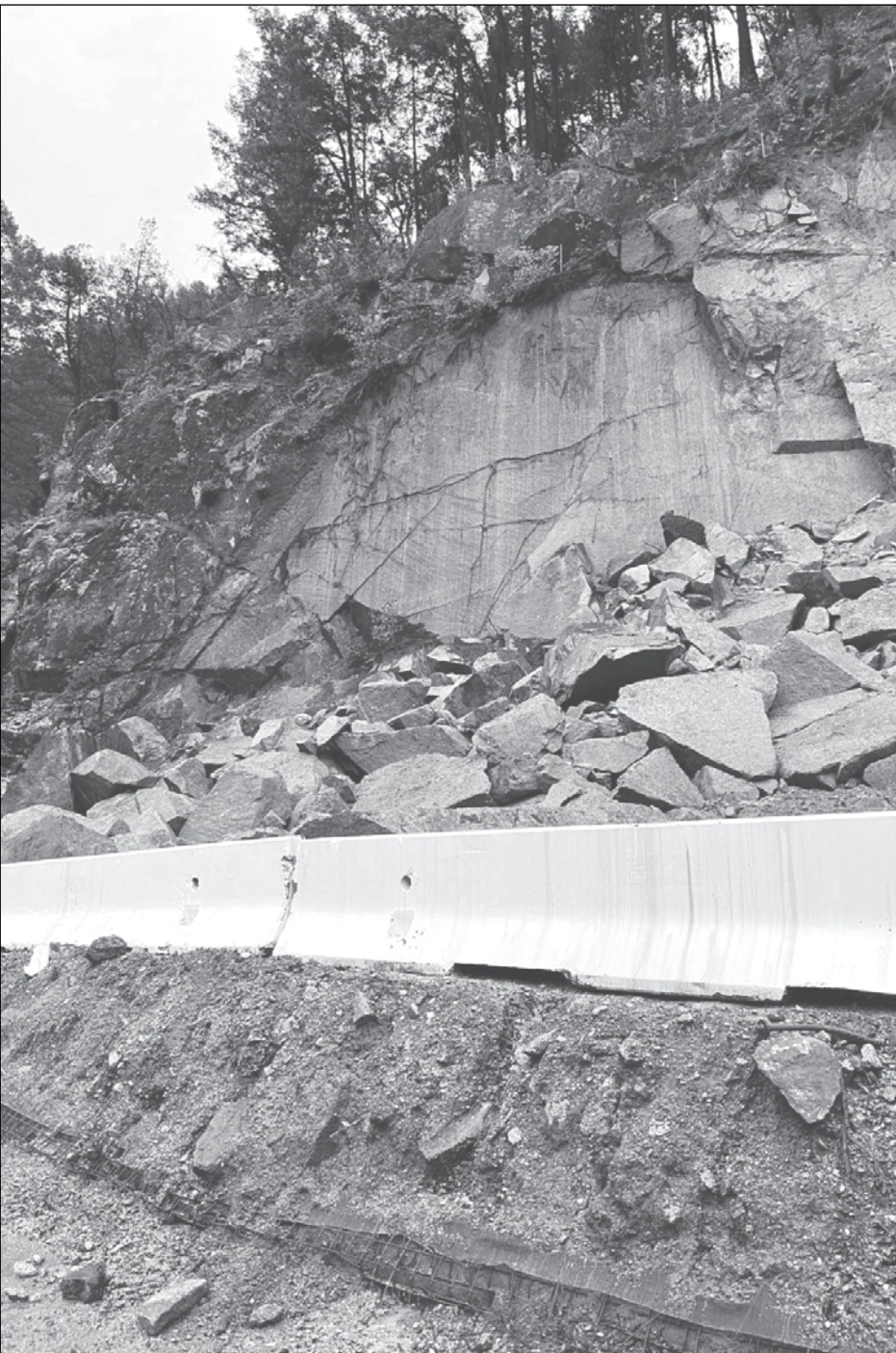
The rockslide that delayed Route 70’s opening has now been cleared. Photo courtesy of Caltrans
