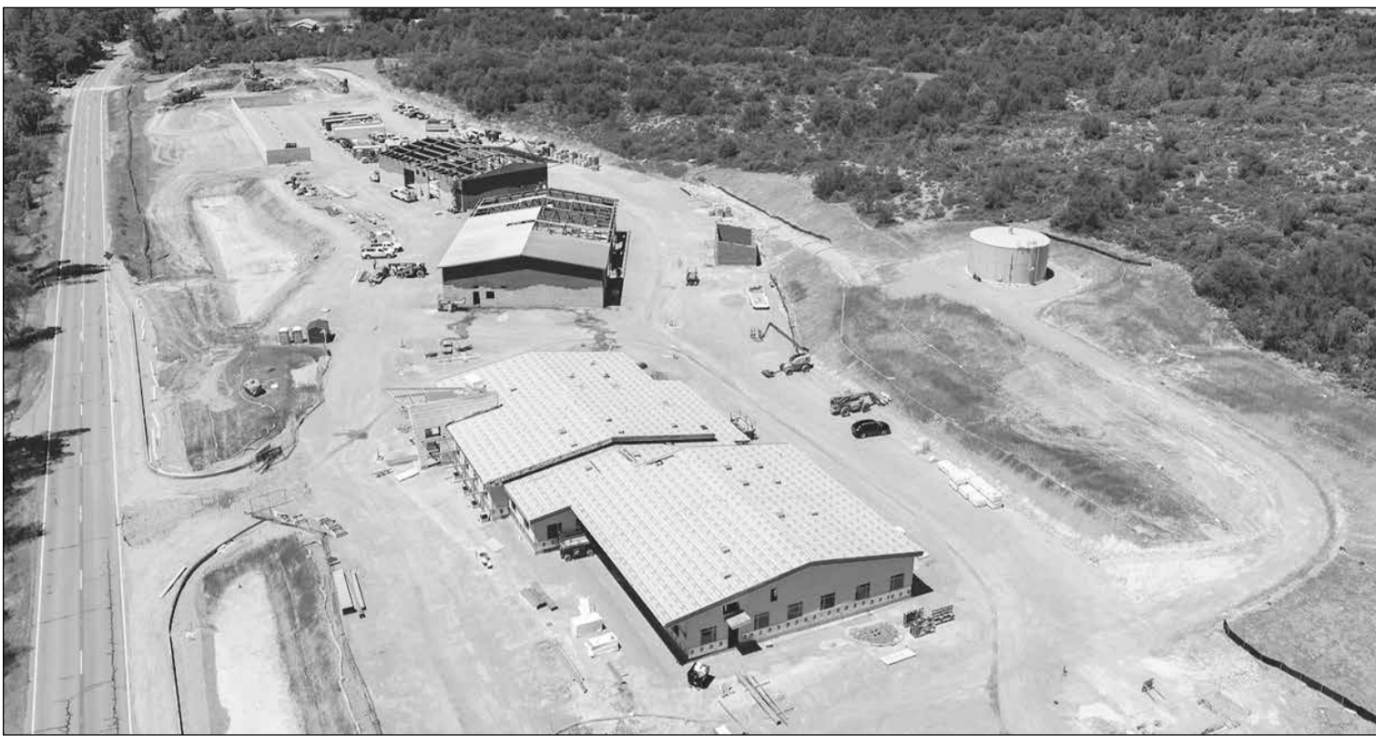
Work continues on Yuba Water Agency's new facilities on Marysville Road. All five buildings on the property are taking shape and work is on schedule. Photo courtesy of Yuba Water Agency
