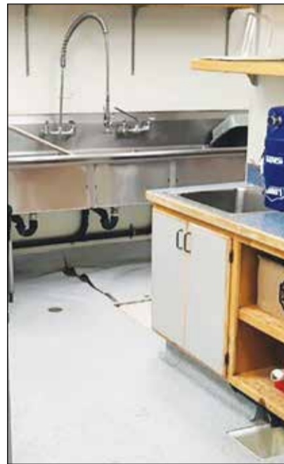
The linoleum in the community center kitchen was beginning to ripple and become unsightly. Photo provided by Paul Breitag
